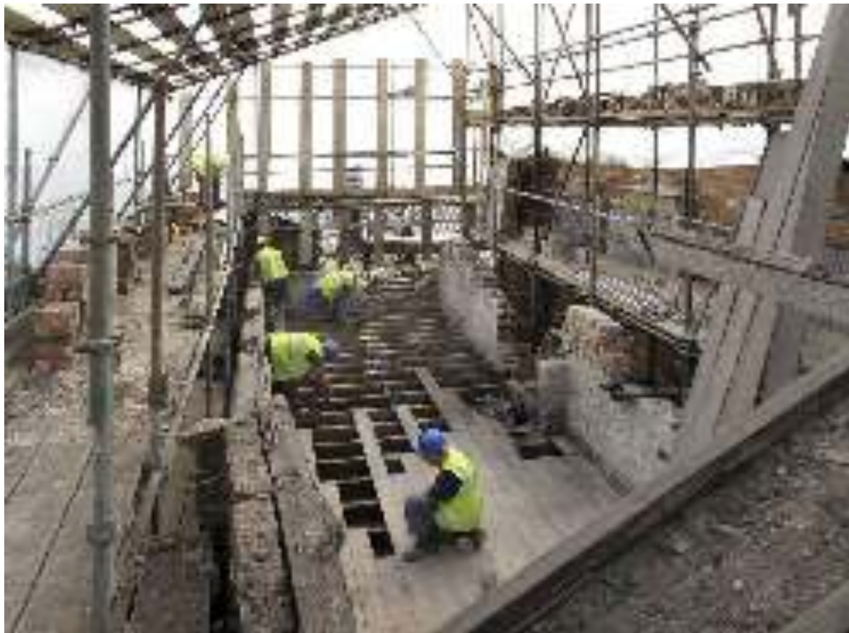
J W Evans and Sons Ltd silverworks undergoing major conservation works prior to opening to the public by English Heritage as a visitor attraction.
