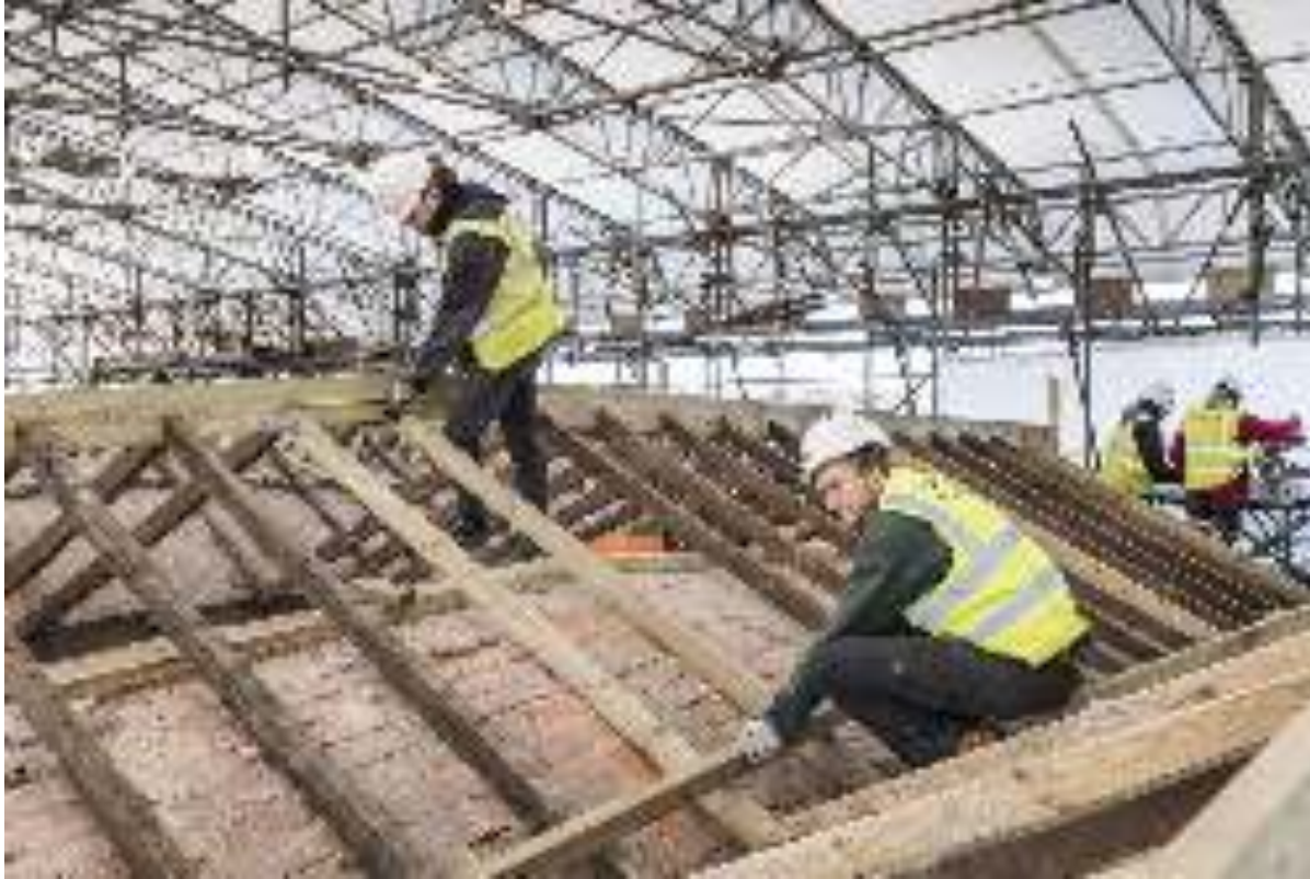
Shrewsbury Flaxmill Maltings, Ditherington, Shrewsbury, Shropshire. Prince's Foundation placements Tom Mott and Sam Rowland-Simms working with Croft Building & Conservation Ltd on repairs to the roof over the main mill
