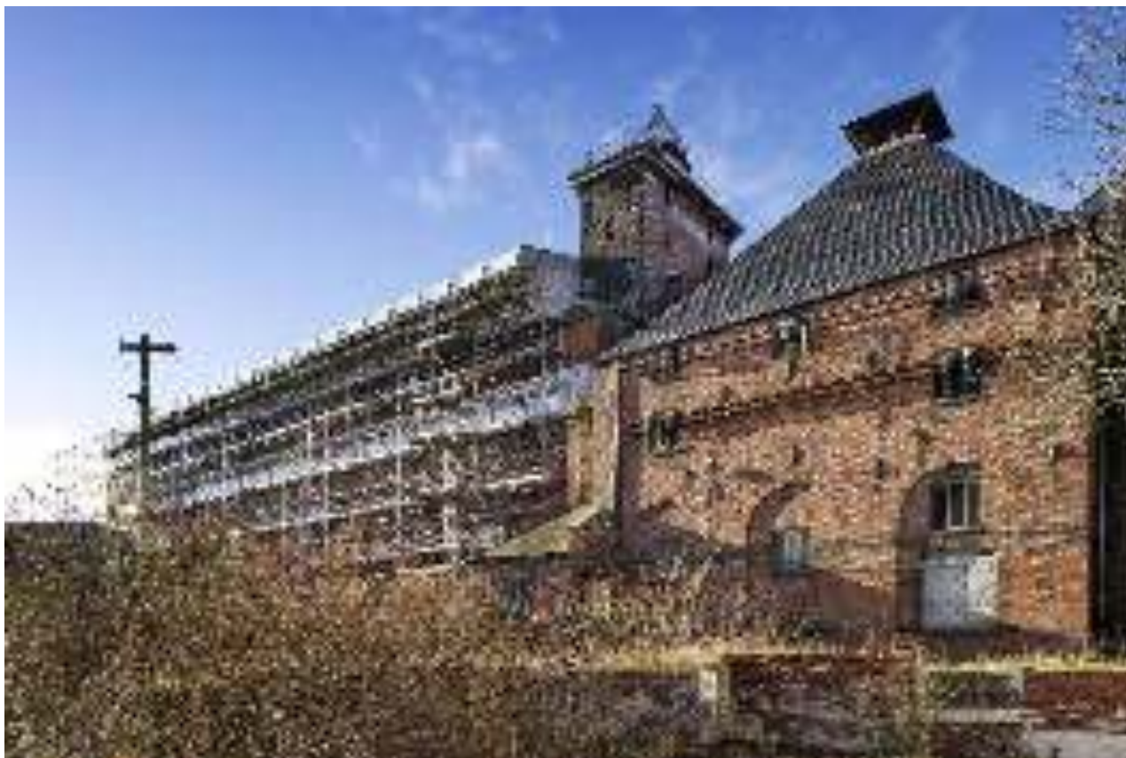
Shrewsbury Flaxmill Maltings, Ditherington, Shrewsbury, Shropshire, the world's first multi-storeyed, iron-framed building, dating from 1797. Spinning mill and kiln, view from north east.
