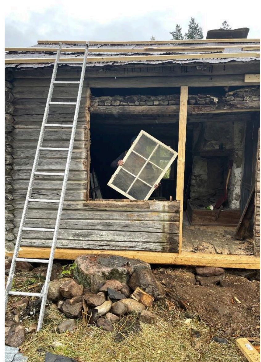
Restoration at Asnes, Finnskogen. Photo: Tove Elise Ihler, The Directorate for Cultural Heritage Research
